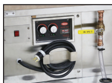
Control Panel, Well Drain
