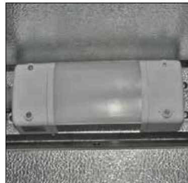
LED light fixture
