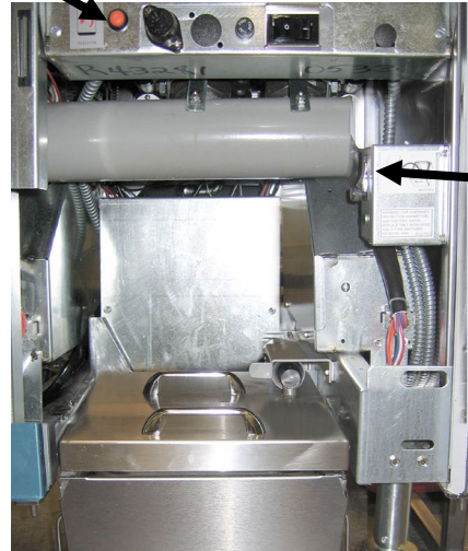
Melting unit power switch
